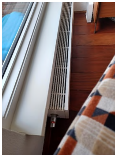
Convactor in woning (boven de vloer)
